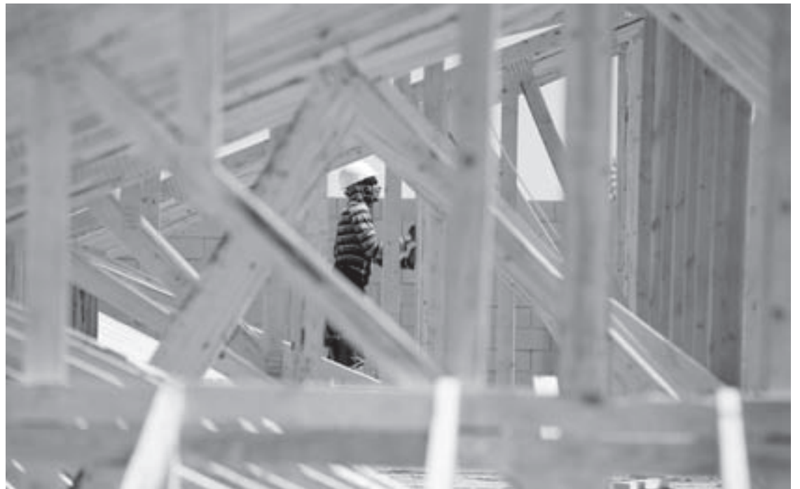
A worker helps to frame a new home at a housing tract in Las Vegas. A big jump in apartment construction in the Midwest and South boosted the pace of homebuilding in November, marking a solid bounce back after tumbling in October. (AP Photo/John Locher)
